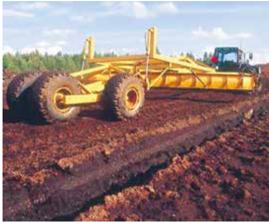
FIGURE 10. Profiling/grading blade finishes the field surfaces to an even shape in both preparation and production stages of the peat production area's life cycle (Vapo Oy).
