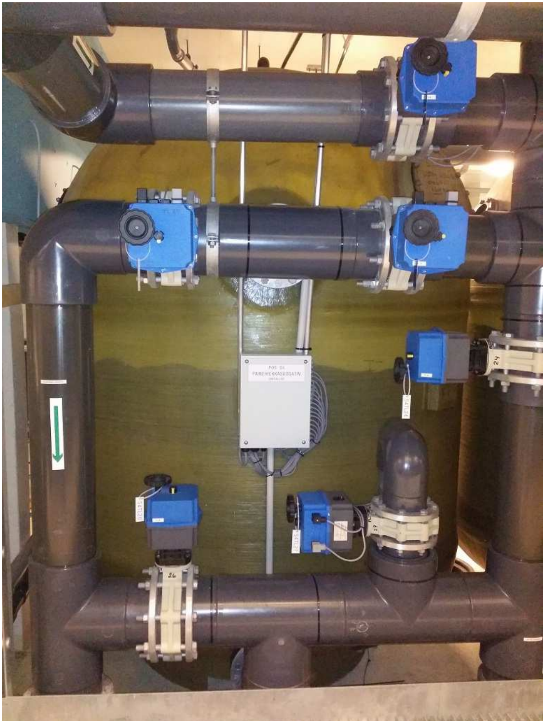
Figure 5 Large sand filter (behind) and blue valves connecting to it.
