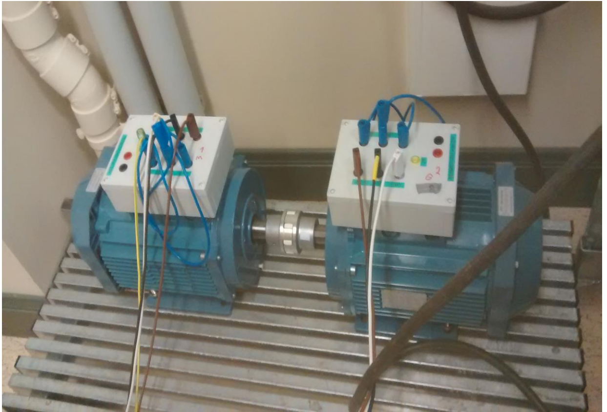
Fig22: Motor and generator coupling
